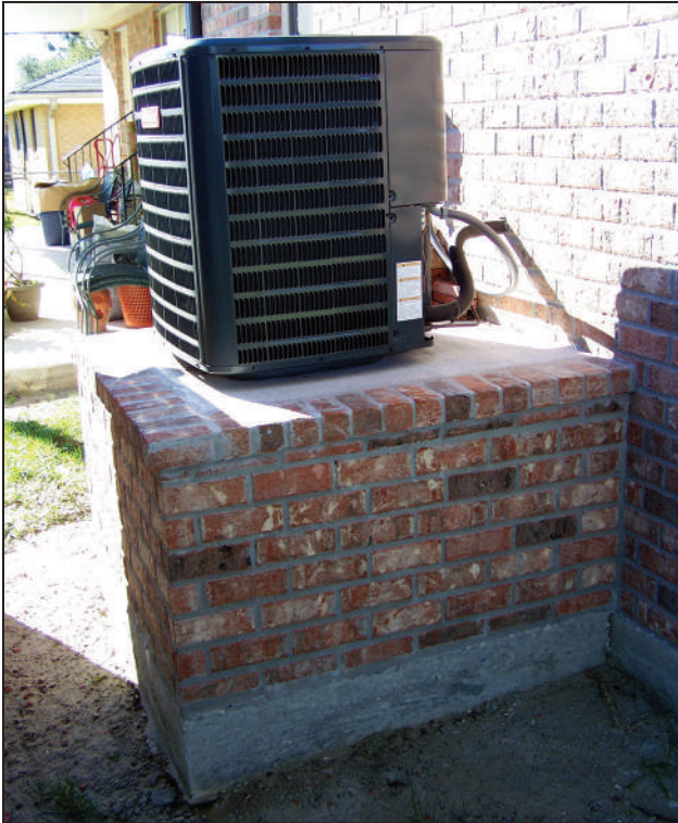
Figure 3-1. Air conditioning compressor elevated on a pedestal.
