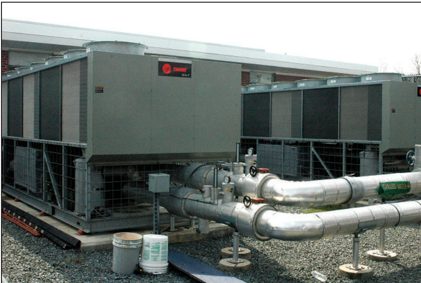
Figure 5-3. Air-Cooled rooftop chiller in Georgetown, Delaware.
