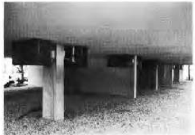
Figure 4.49. Elevated Condenser Units
