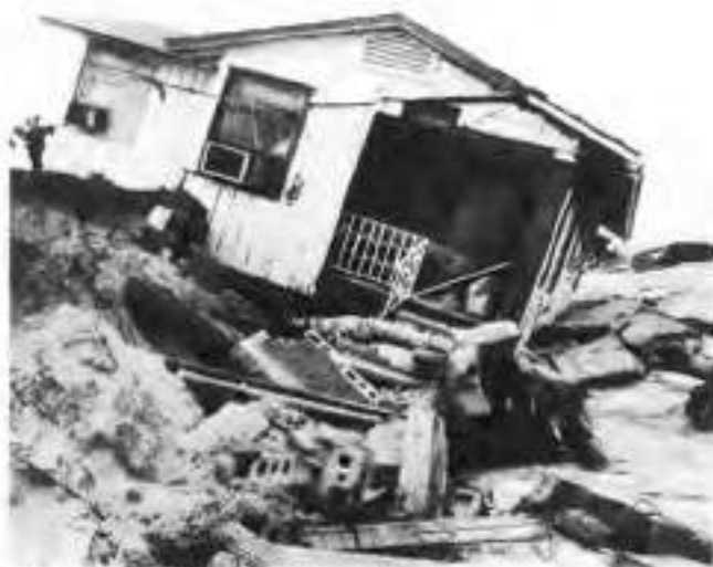
Figure 2.3. Erosion Caused This Foundation to Collapse.
