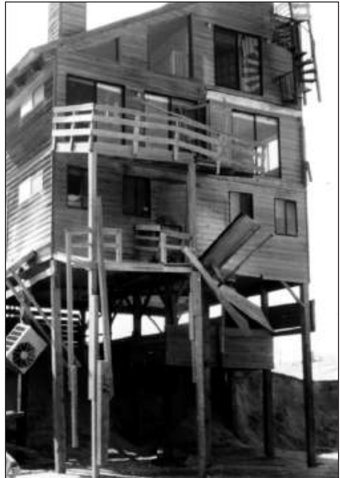
Figure 2-3. Although this house seems to have lost only several decks and a porch during the March 1989 nor'easter, the loss of supporting soil due to long-term erosion left its structural integrity in question following successive storms
