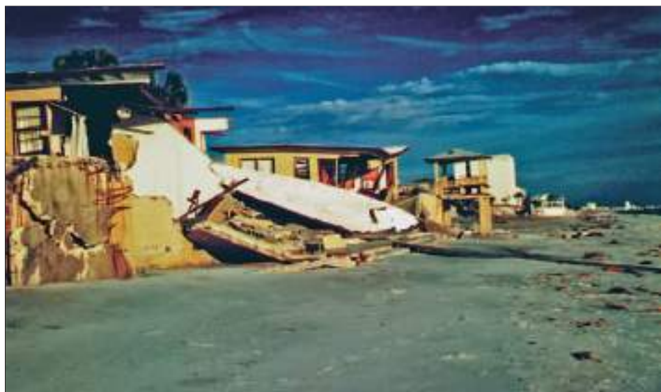
Figure 3-45. Failure of seawall in Bay County, FL, led to undermining and collapse of the building behind the wall (Hurricane Opal, 1995)
