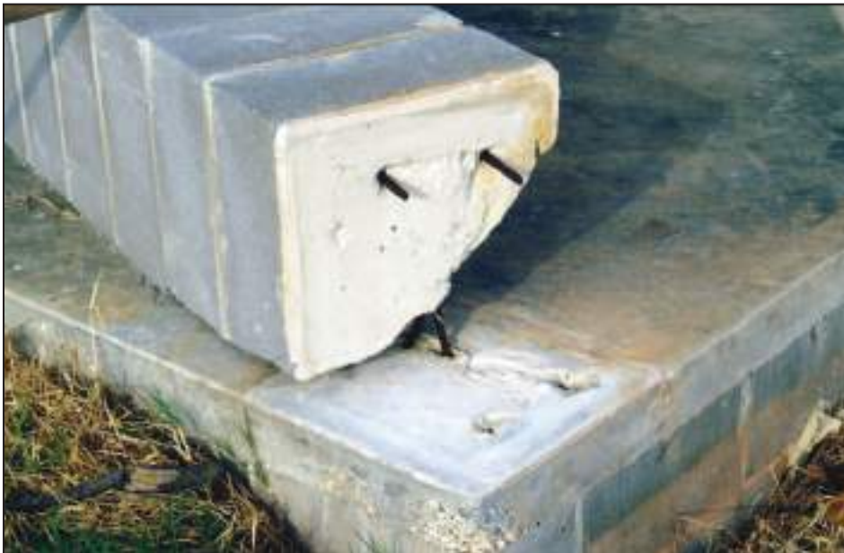
Figure 2-18. Failed masonry column connection, Hurricane Katrina (Jackson County, MS, 2005)
