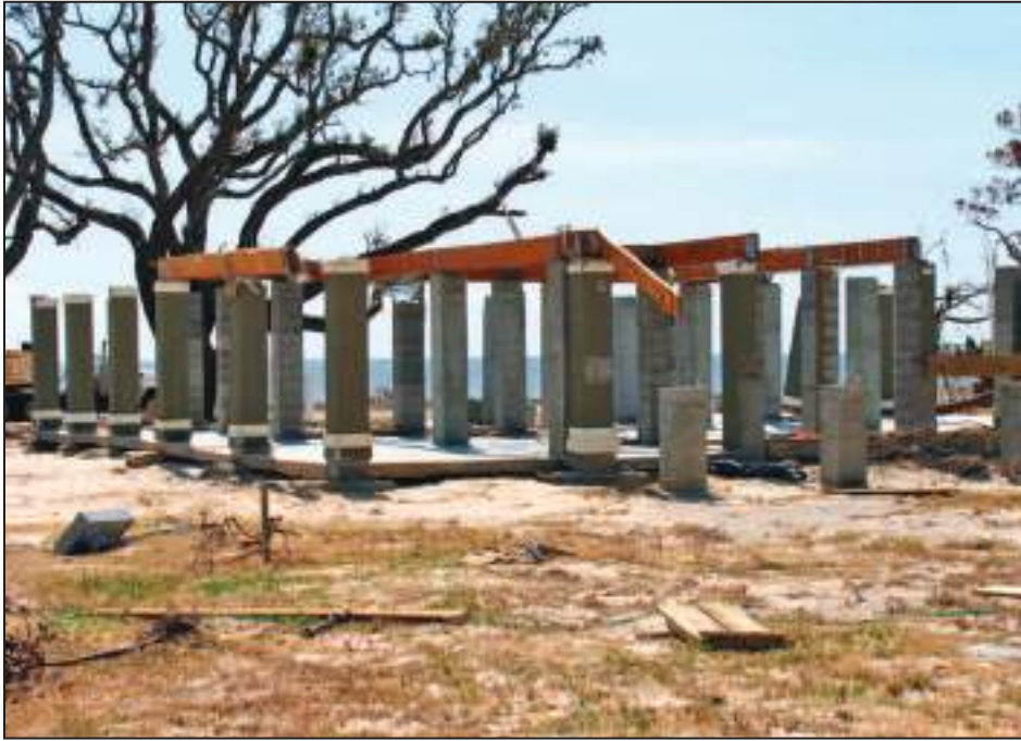
Figure 2-5. This elevated house atop a masonry pier foundation was lost, probably due to waves and storm surge reaching above the top of the foundation, Hurricane Katrina (Long Beach, MS, 2005)
