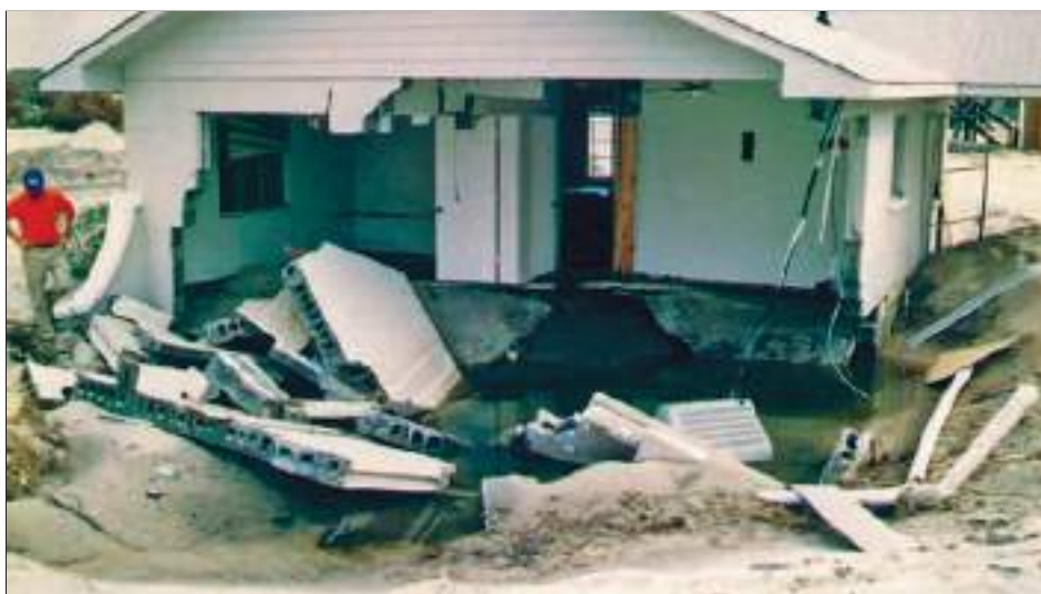
Figure 2-13. Extreme case of localized scour undermining a Zone A continuous perimeter wall foundation located several hundred feet from the shoreline, Hurricane Fran (Topsail Island, NC, 1996)
