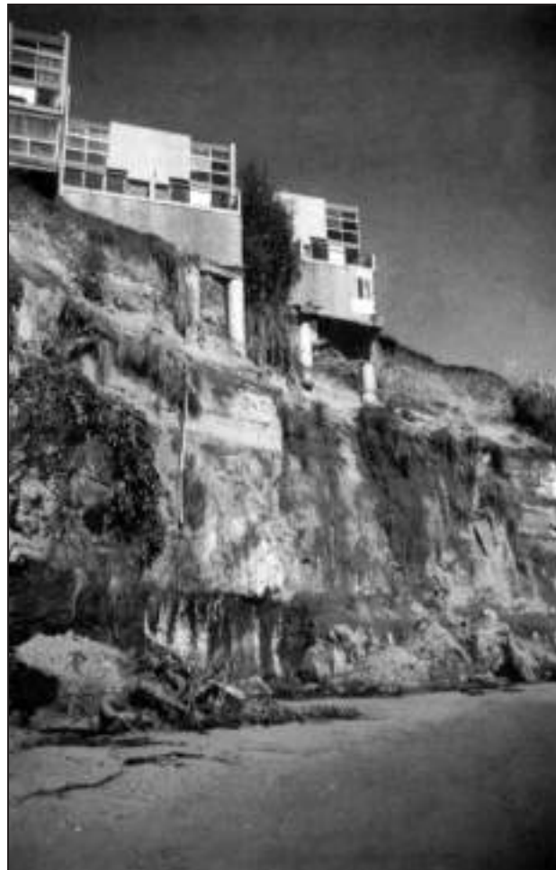
Figure 3-37. Bluff failure by a combination of marine, terrestrial, and seismic processes led to progressive undercutting of blufftop apartments at Capitola, CA, where six of the units were demolished after the 1989 Loma Prieta earthquake SOURCE: GRIGGS 1994, JOURNAL OF COASTAL RESEARCH , USED WITH PERMISSION
