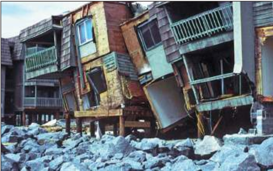
Figure 4-23. Damage to buildings sited behind a rock revetment close to an eroding shoreline at Garden City Beach, SC (Hurricane Hugo, 1989)
