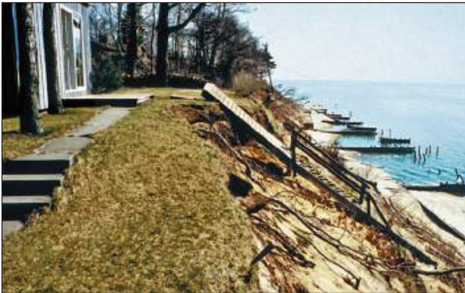
Figure 2-7. Erosion along the Lake Michigan shoreline at Holland, MI, resulting from high lake levels and storm activity (August 1988)
